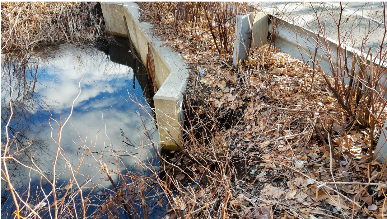
The knotweed surrounding this culvert is contributing to the loss of soil, which threatens both the roadway and the guardrail.
